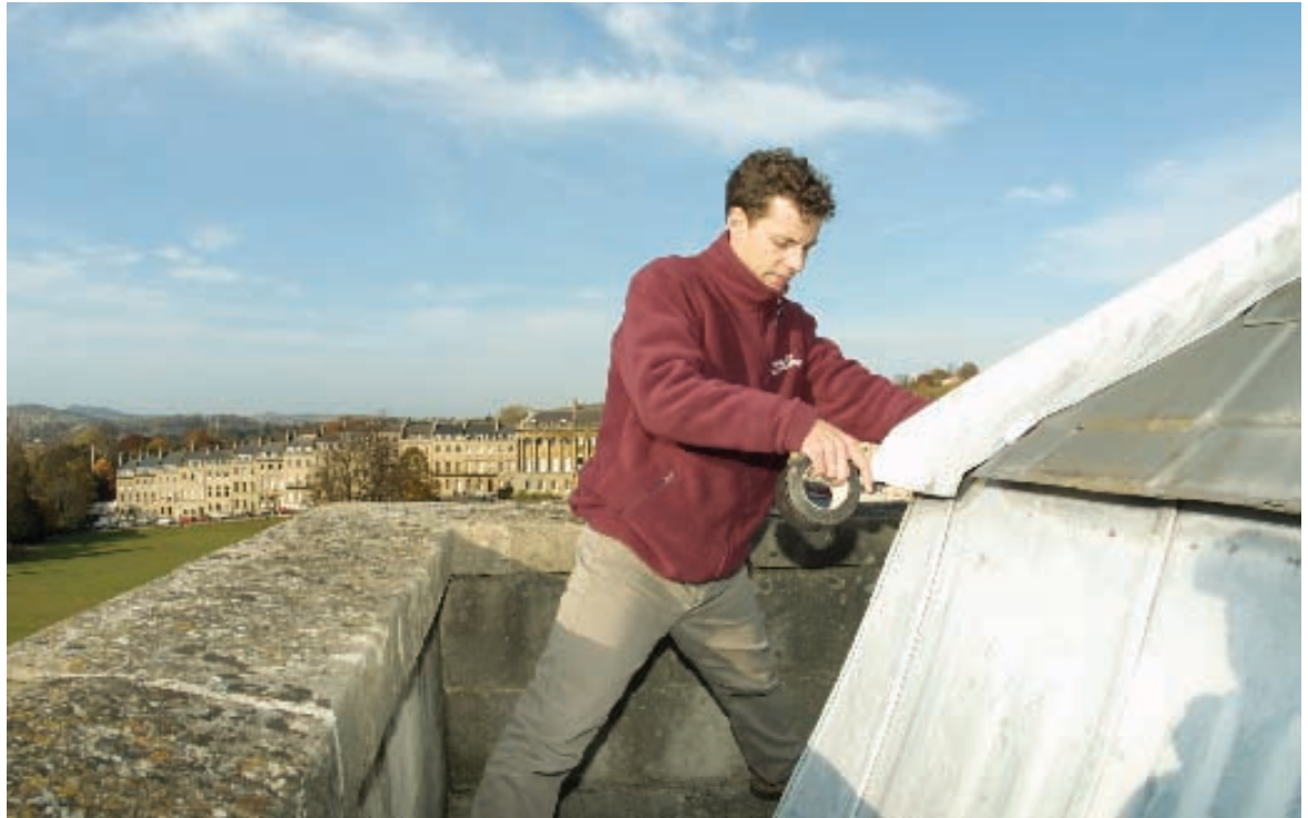
An MoH inspector making temporary flashband repairs at the Royal Crescent, Bath
