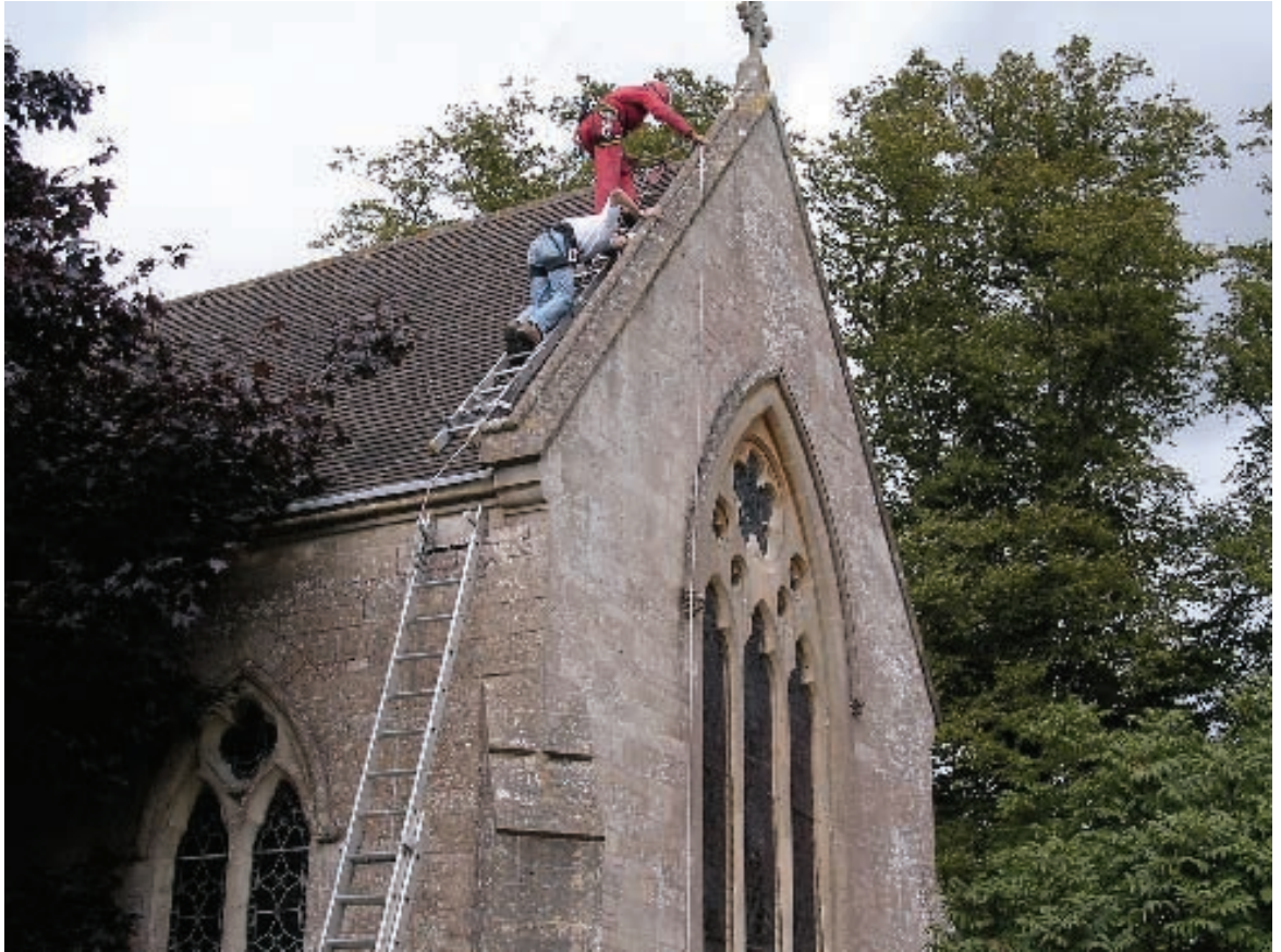
Maintain our Heritage inspectors using roped access (provided by Wall Walkers) on the church of St John the Baptist, Shipton Moyne, Gloucestershire
